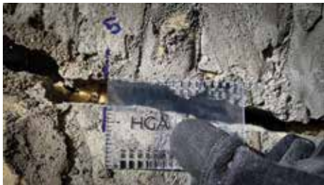
Monitoring cracks at masonry
