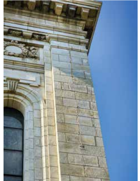
Exterior stone cracks
